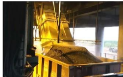
Automatic Wagon Loading System
