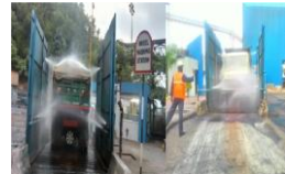
Automatic Wheel Wash System
