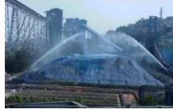
Realtime dust monitoring and Automated Sprinkler System
