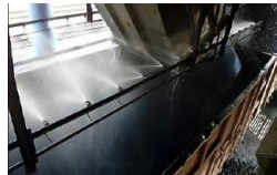
Dry Fog Dust Suppression at Wagon Loading System
