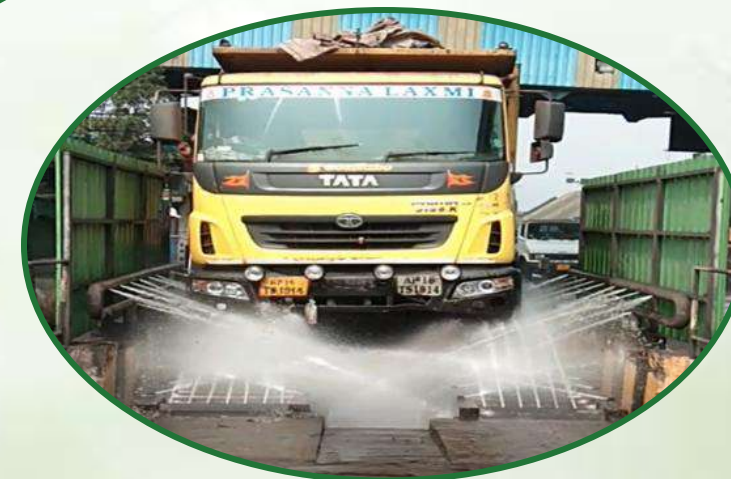
Truck Tyre Washing Facility
