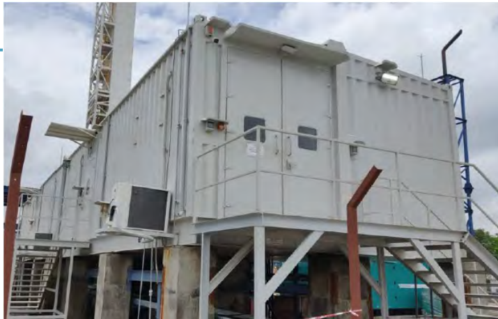
Siemens A/c Tata Steel, West Bokaro
