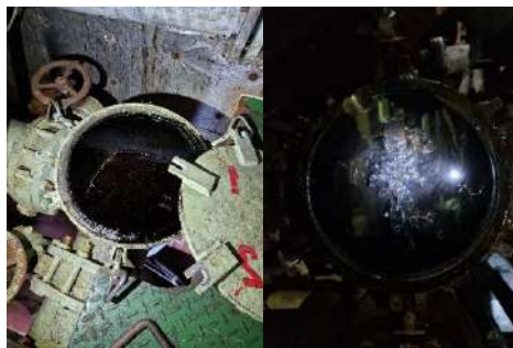
Bilge and ballast eductor suction filter and Fire & Bilge pump suction filter found with oil.
