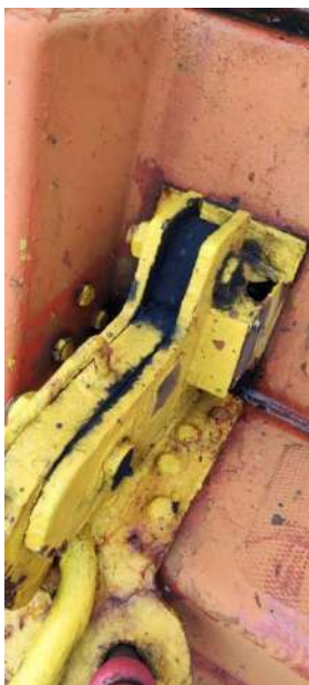
Free fall lifeboat hook securing base corroded and holed
