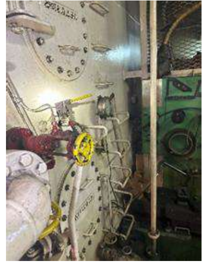
Quick closing valve spindle missing
