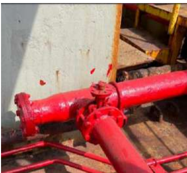
Broken Fire line V/V
