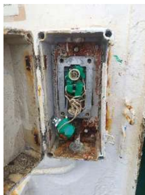
Sludge P/P Remote St./Stp. Switch Defective
