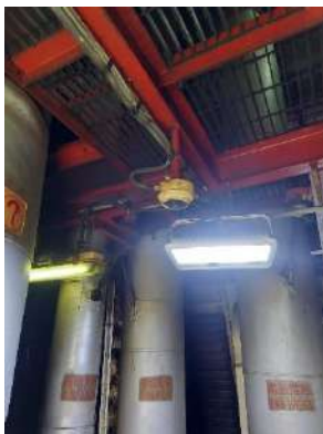
Damaged Fire Detector
