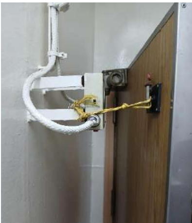
Accom. fire doors tied up.
