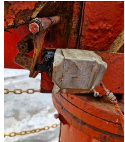
Limit switch for davit non operational
