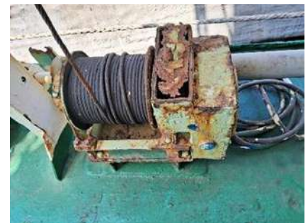
Corroded Accommodation winch
