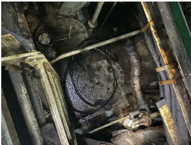
Unauthorised snap coupling fitted on sludge pump suction pipe
