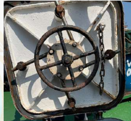
Damaged booby Hatch packing
