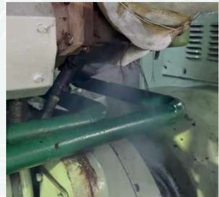
Exhaust leakage from A/E
