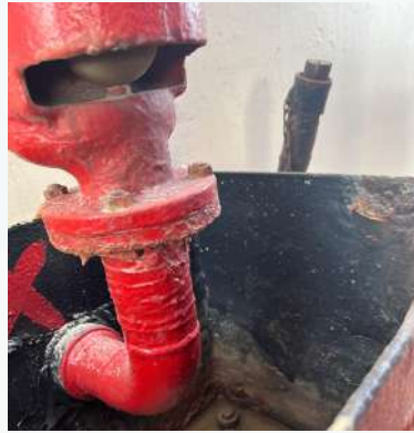
Damaged air vent
