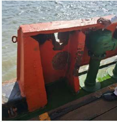
Hole in Bulwark
