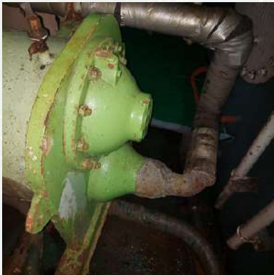
Devcon putty on AC condenser sw cooling line
