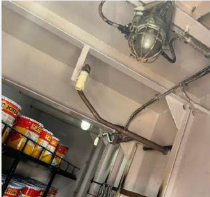
Paint room water sprinkler closed with tape.
