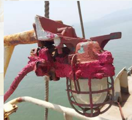
Embarkation light not working and damaged
