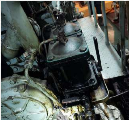
Leaking Fuel Oil from AE
