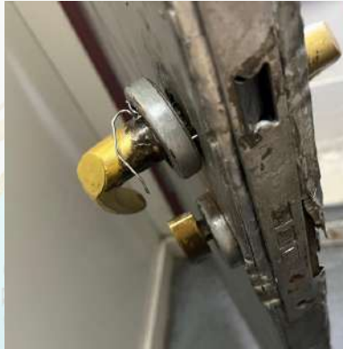
Damaged engine room door
