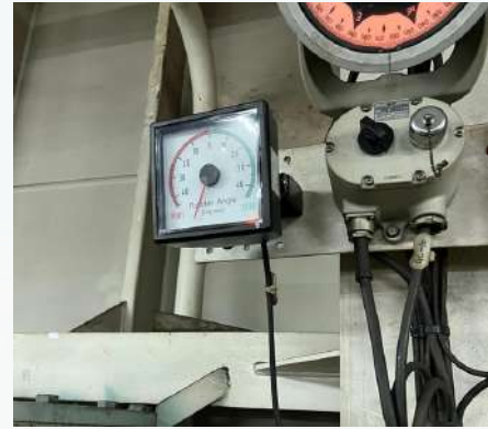
Defective Rudder angle indicator
