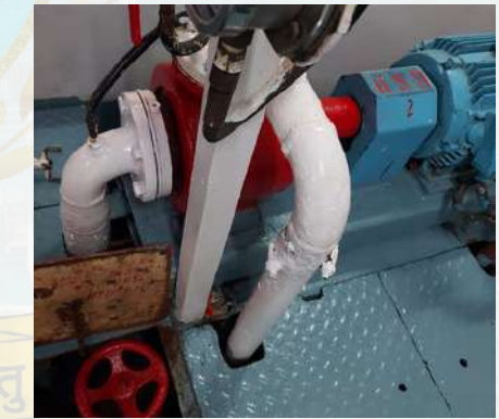
Fire pump outlet pipe leaking and temporarily repaired
