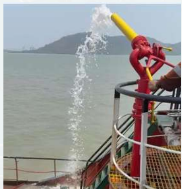
Ineffective foam monitor
